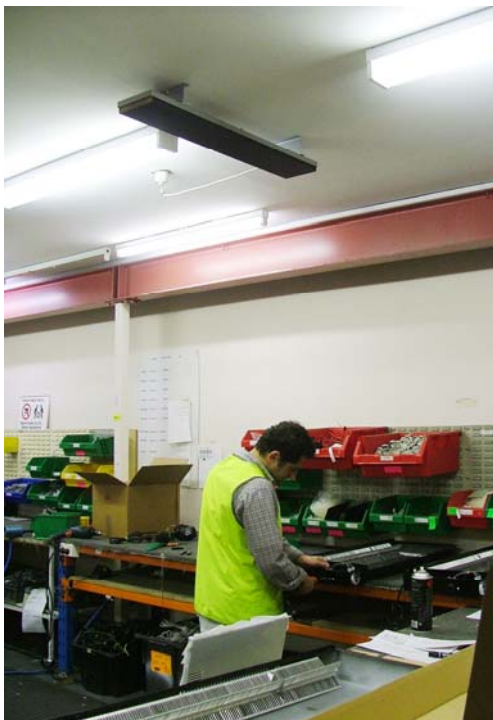
Individual workstation spot heating example in factory
